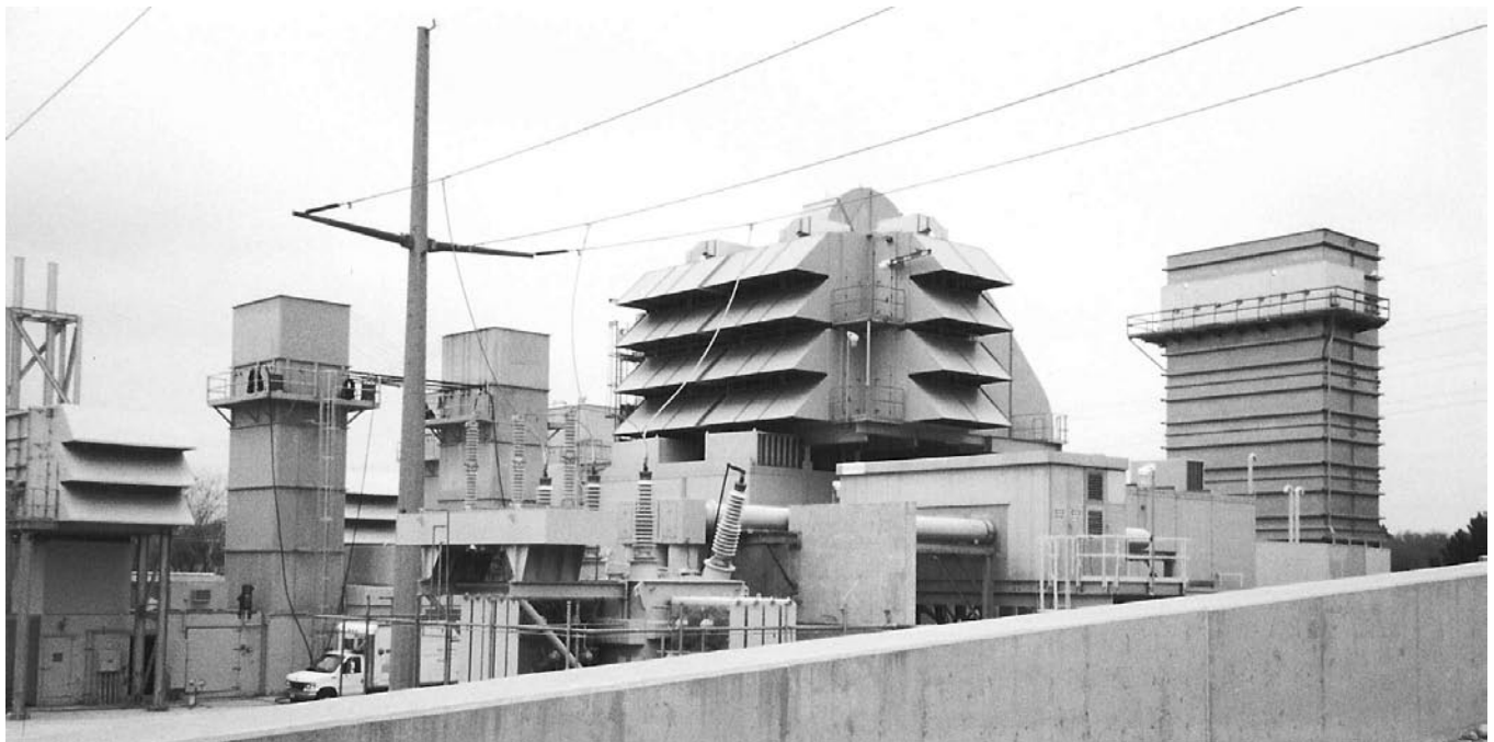
Fig. 1— An aero-derivative combustion turbine (unit with dual stacks) rated at 50 MW next to an industrial combustion turbine rated at 120 MW. Hooded assemblies are combustion air inlets. Vertical rectangular stack assemblies are turbine exhaust silencers venting to atmosphere.
