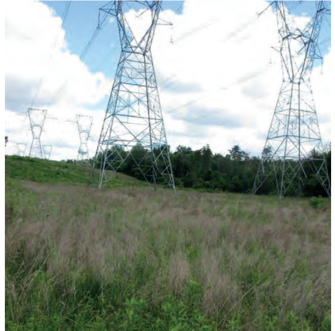
figure 2-2 | High Voltage Transmission Lines
