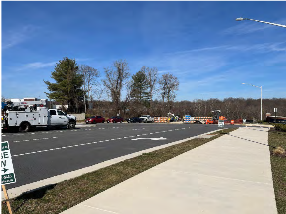
Photograph # 24 – Active roadway construction occurring immediately northwest of study area at existing terminus of Annapolis Way (3/1/2024)
