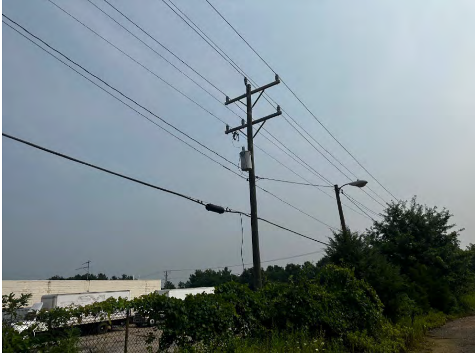
Photograph # 13 - Pole mounted transformer on eastern property line (7/13/2023)
