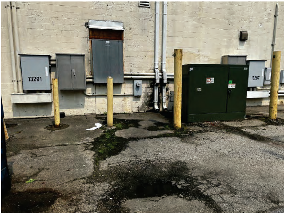
Photograph # 12 - Utility connections for onsite buildings (typical) (7/13/2023)
