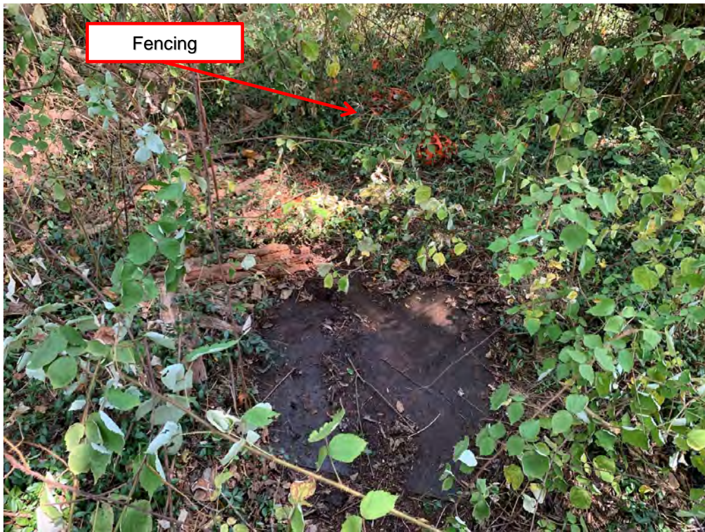
Photograph 14: Potential Covered Well Shaft. Note orange fencing. View north (MN 8/29/2024).
