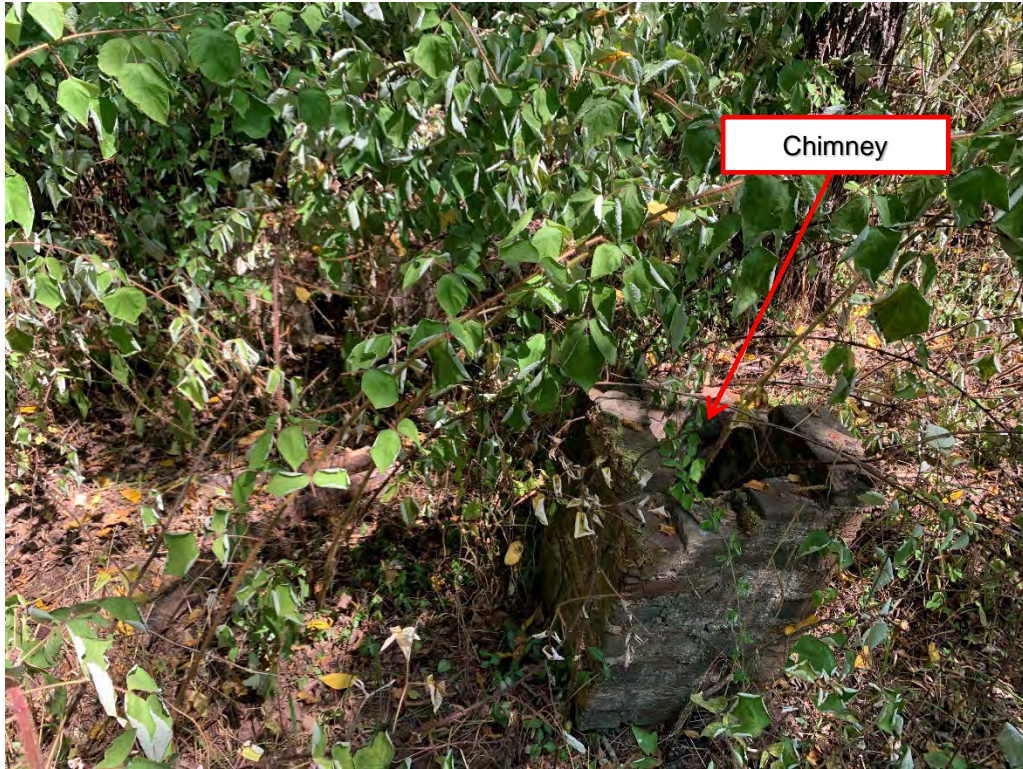
Photograph 12: Chimney Fall Near East Foundation. View north (MN 8/29/2024).
