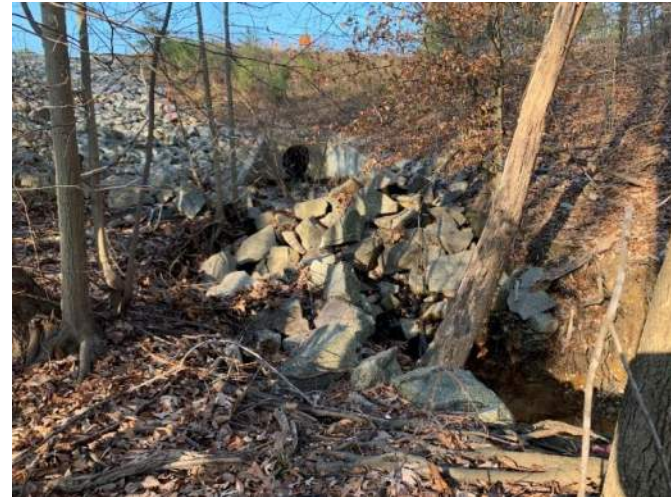
Photo #64: Representative Photo of system PG (R3) looking upstream starting at a culvert under Four Seasons Drive. Date: December 10, 2020
