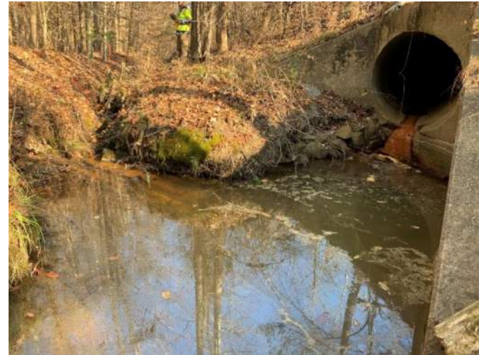
Photo #68: Representative Photo of system PI (R3) looking upstream with the culvert going under I-95. Date: December 10, 2020
