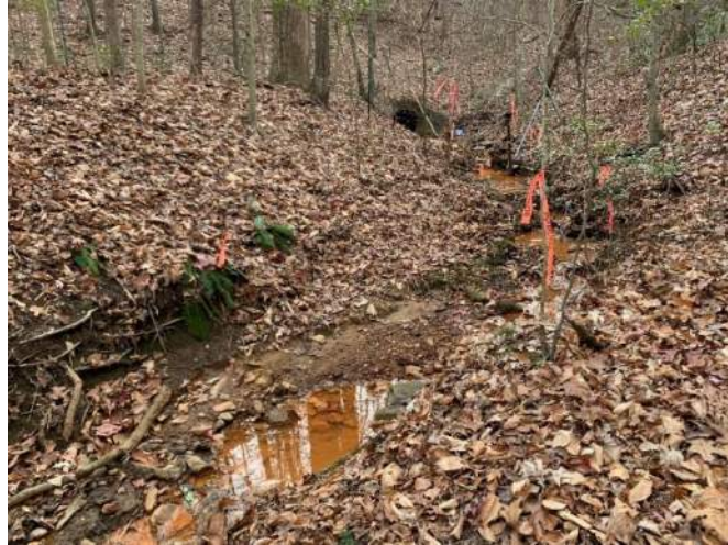
Photo #79: Representative Photo of system W (R3) looking upstream with the culvert going under I-95. Date: December 9, 2020
