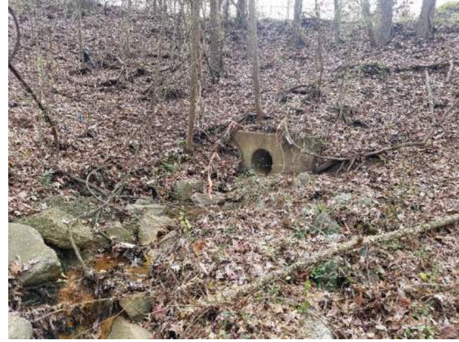
Photo #18: Representative Photo of system DA (EPH) looking upstream starting at a culvert that goes under Old Stage Road. Date: December 9, 2020
