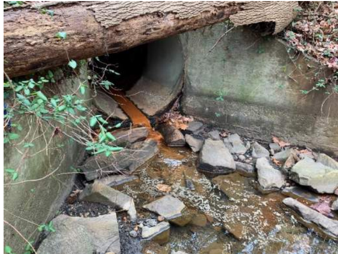
Photo #31: Representative Photo of system H (R4) looking upstream starting a culvert that goes under I-95. Date: December 22, 2020
