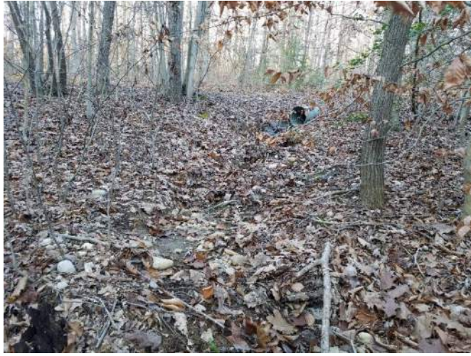
Photo #25: Representative Photo of system F (EPH) looking upstream starting at a pipe going under the sewerline easement access road. Date: December 9, 2020
